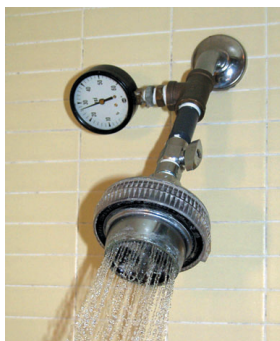
Figure 3. Pressure at 28 psi as lone fixture
