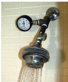
Figure 4. Pressure at 14 psi with two other showers running
