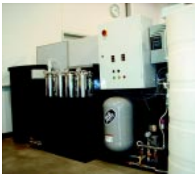
Water recycling system
