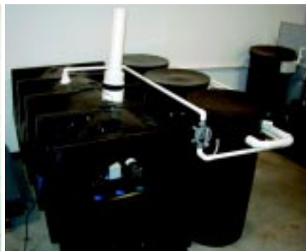
Separation/composting, greywater treatment and ozone contact tanks
