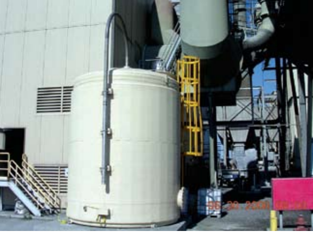
Small industrial RO installation
