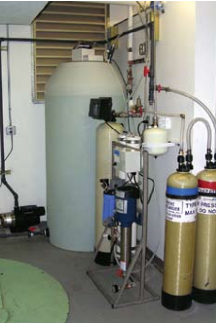
Small commercial RO installation
