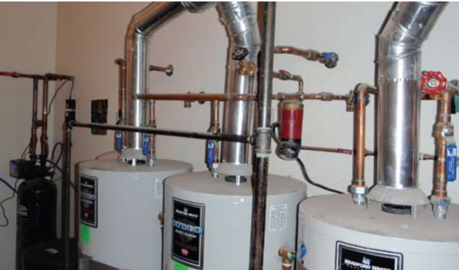
Mechanical room with water heaters, softener and recirculation pump (red cylinder connected to the copper piping)
