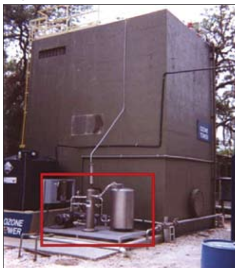
Figure 4. Gas injection and degasification skid
